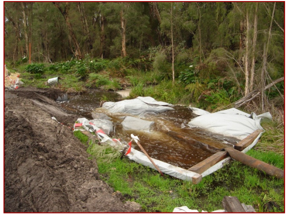
Watercourse crossing flume to maintain downstream flow regime with erosion prevention blanket
