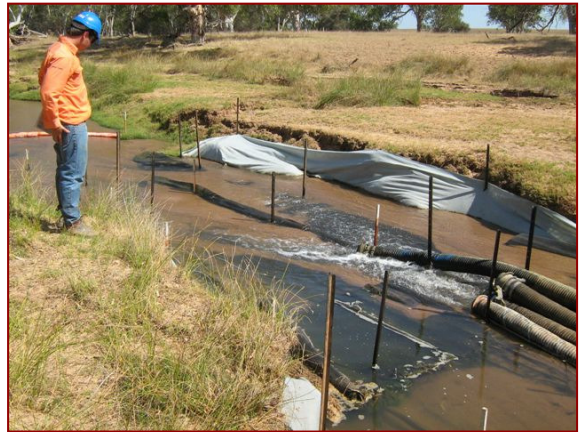
Watercourse crossing flume to maintain downstream flow regime with erosion prevention blanket
