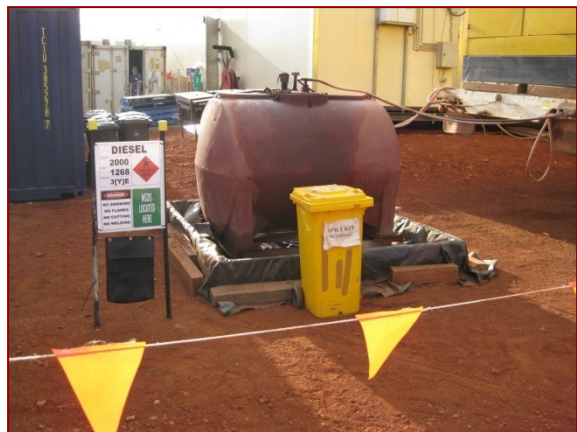
Bunded generator set fuel tank and spill kit
