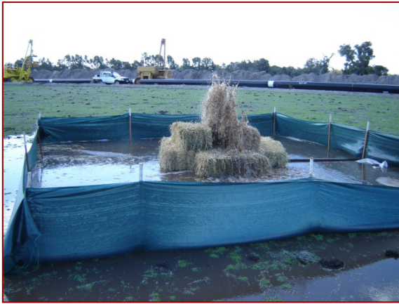
Disposal of water dewatering discharge onto paddock through hay bales and sediment trap
