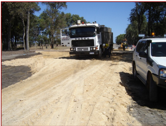
Limestone hardstand at property boundary to prevent affected soil transfer through adherence to vehicles
