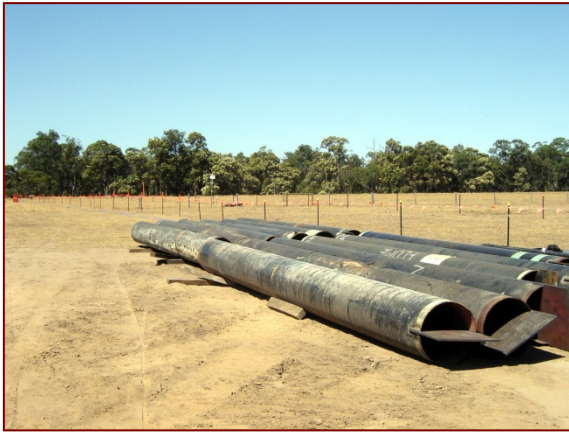
Horizontal directional drilling entry point at Murray River, approximately 200 m from river bank (in background)
