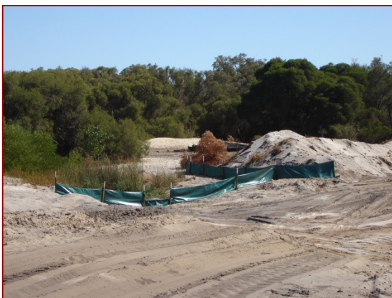
Watercourse crossing sediment trap
