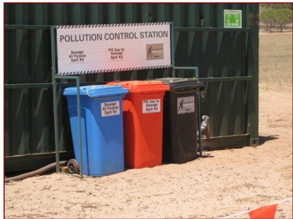
Pollution control station with spill kits for package wastewater treatment plant
