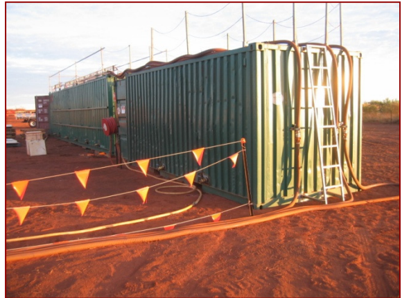
Package wastewater treatment at camp sites
