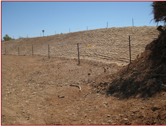
Sand and cement filled sandbags used for watercourse bank stabilisation, fenced to prevent stock damage
