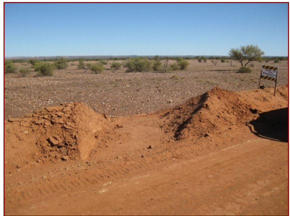
Topsoil stockpile adjacent to CROW source area with drainage slot to prevent water ponding
