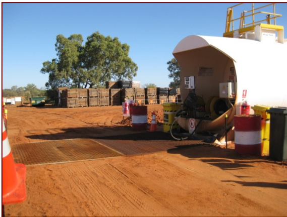
Multiple fuel spill capture tanks and grate at bulk refuelling station
