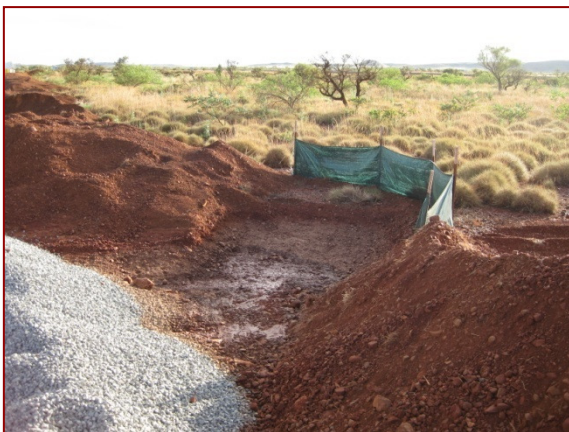
Sediment trap for surface drainage discharges from campsite area
