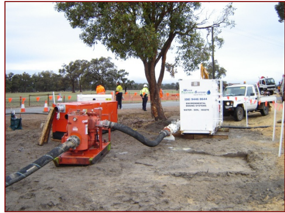
Automated pH correction plant for dewatering effluent from acid sulphate soil area prior to disposal
