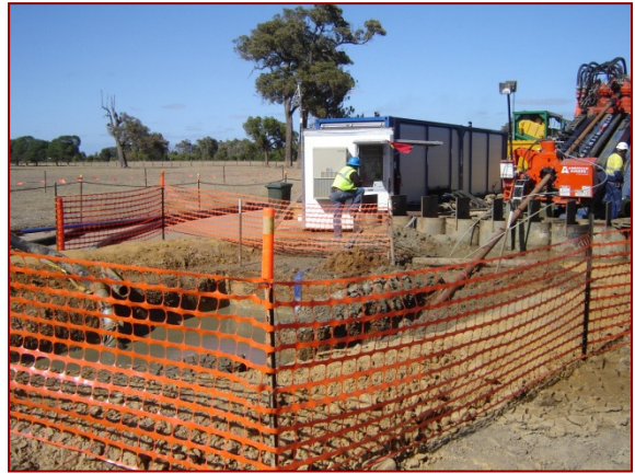
Horizontal directional drilling entry point at Murray River looking away from river
