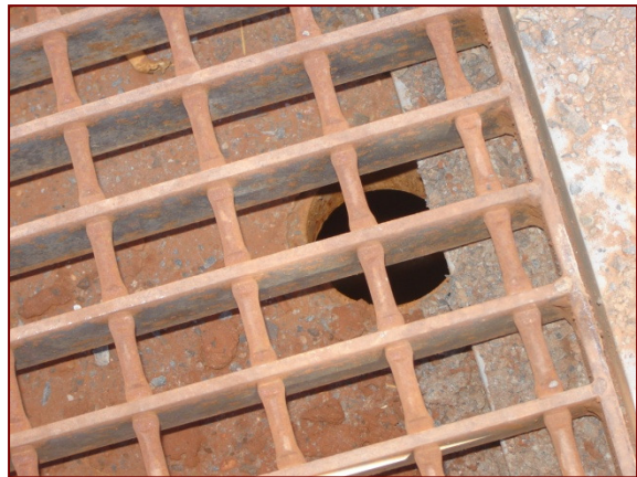
Drain hole in base of fuel spill capture tank leading to 200 L recovery drum
