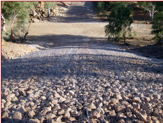
Rock armouring with mesh anchoring for watercourse bank stabilisation on long steep bank (Wooramel River)
