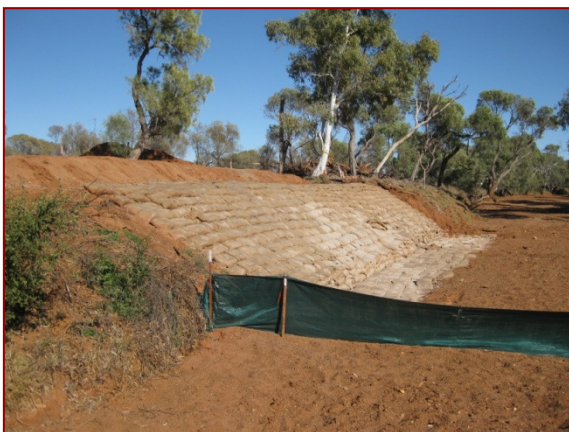
Sand and cement filled sandbags bank stabilisation under construction with temporary silt fence
