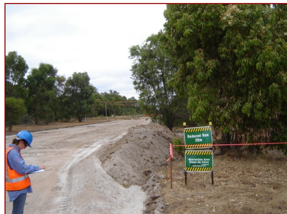
Reduced CROW width associated with entry to DRF area
