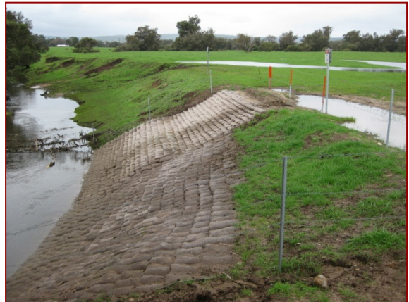
Sand and cement filled sandbags used for watercourse bank stabilisation, fenced to prevent stock damage
