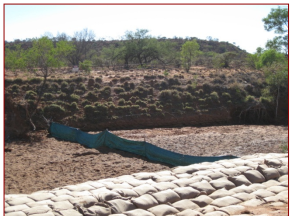
Sand and cement filled sandbags bank stabilisation under construction with temporary silt fence
