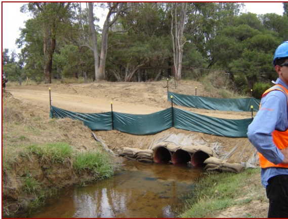
Watercourse crossing flume with high flow sediment traps
