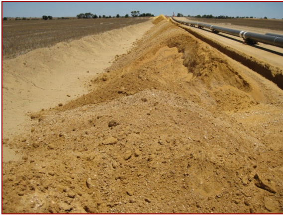
Topsoil stockpile adjacent to CROW source area (on left), separate from trench spoil stockpile (centre)
