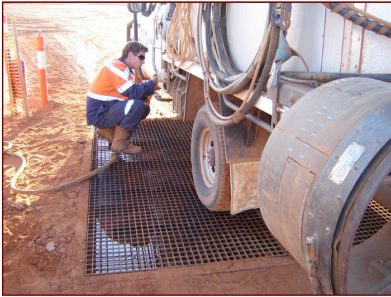
Fuel spill capture tank and grate beneath filling point (note captured liquid below grate)
