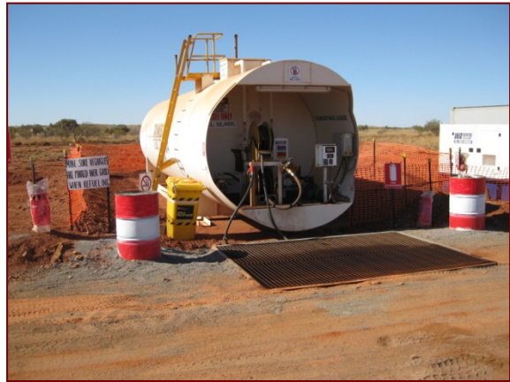
Fuel spill capture tank and grate at bulk refuelling station
