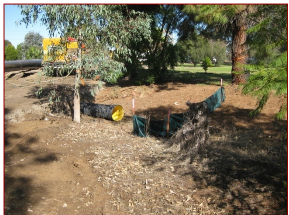
Watercourse crossing flume with sediment trap
