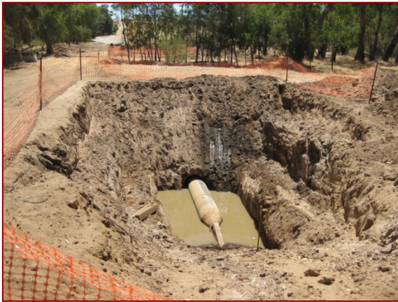
Horizontal directional drilling exit point at Caren Caren Brook looking across watercourse
