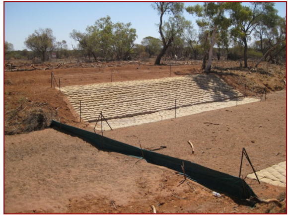
Sand and cement filled sandbags used for watercourse bank stabilisation, fenced to prevent stock damage
