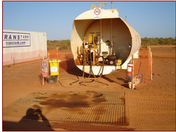
Fuel spill capture tank and grate at bulk refuelling station (note fuel spill staining)
