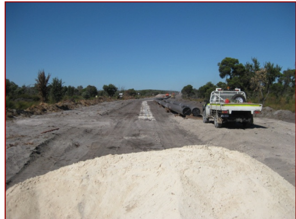
Neutralising agent (aglime) stockpile and dosing laid on pipeline alignment prior to trench excavation
